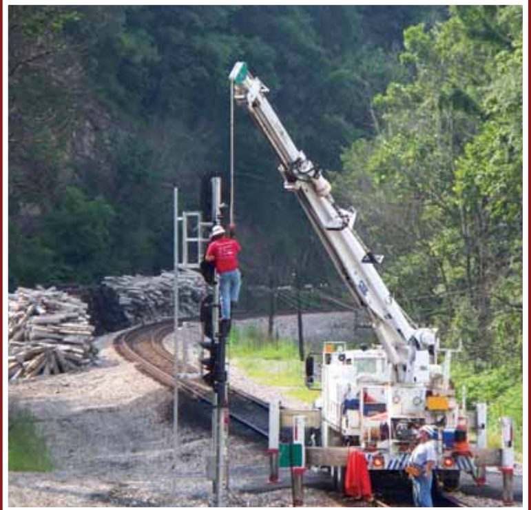
Scott Menix and Tim Cox, both members of Local 136, remove old signals during a cut-in at E.E. Haden. Photo submitted by Local 136 member C.A. Hawkins.
