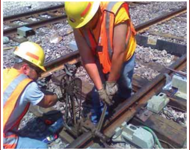
Signal gang foremen Alberto Palencia and Dale Miller, both of local 130, use a hand-crank to install a transducers on a hotbox detector in Pleasant Prarie, Wisconsin, Kenosha Subdivision. Photo submitted by Julio C. Alvarez member of Local 108.
