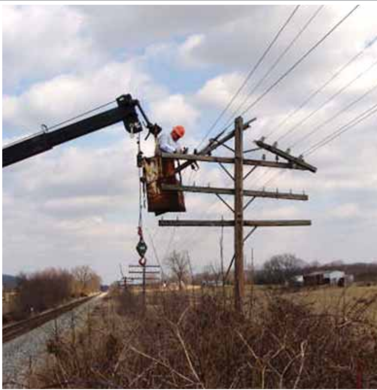
Darrell Ball, Signal Foreman of the CSX Western Region signal construction team 7XJ7, demonstrates the proper use of line blocks during the reconstruction of damaged pole-line on the Main-Line Subdivision in Cave City, Kentucky. Brother Ball serves as Recording Financial-Secretary for Local 158. Photo submitted by Local 136 member Daniel J. Bocook.
