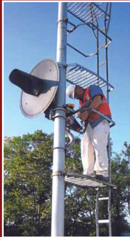
Signal Testman Dennis Roberts of Local 183, tests the relay in a searchlight signal on Metra's Rock Island District, in Blue Island, Illinois. Photo submitted by Kevin Lavin, Local Chairman, Local 183.
