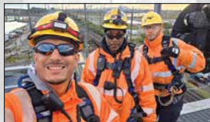
COVER: Brothers from Local 102 hanging signals on the new Portal Bridge in Kearny, New Jersey.
